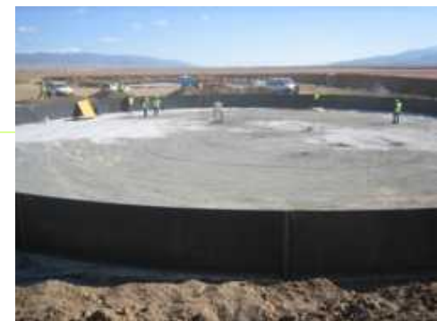
Molten salts tank
